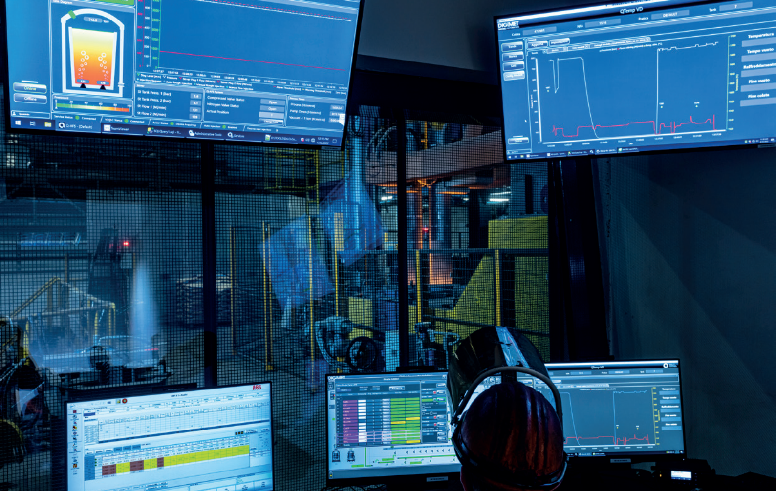
Pulpit with HMI terminals of a state-of-the-art VTD plant (Picture: Danieli)
