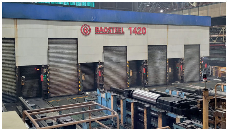
Baosteel's pickling line and tandem cold mill will undergo a major upgrade and modernization (Photo: Primetals Technologies)
