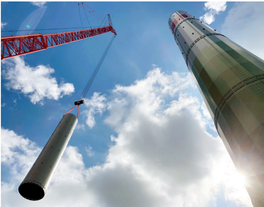
Hybrid steel tower used for a wind turbine from Enercon (Picture: Enercon)
