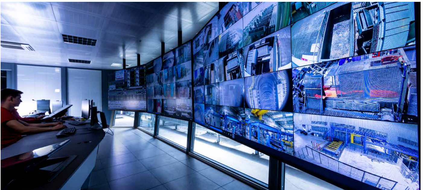
The control room of the QWR quality wire rod mill at ABS (Steel Making segment) (Photo: Danieli)
