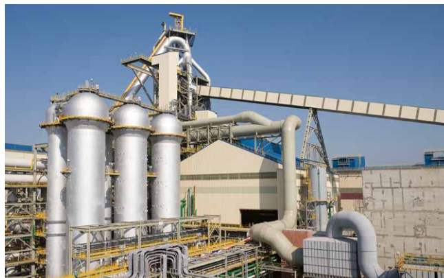
New copper staves will be installed at Dragon Steel Corporation's blast furnace No. 1 (Photo: Primetals Technologies)
