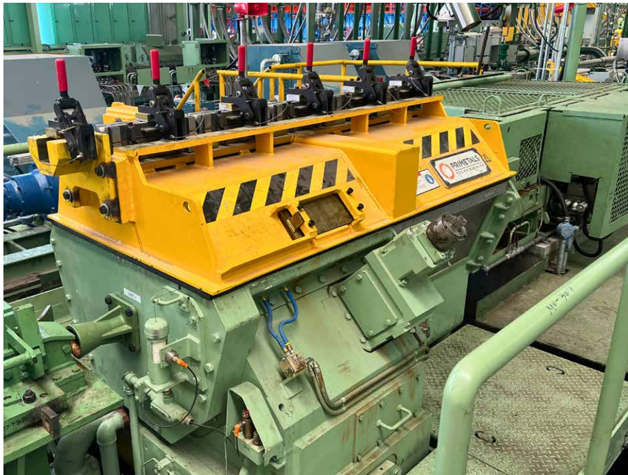
One of the mini-finishing mills installed at Baoshan Iron and Steel (Photo: Primetals Technologies)
