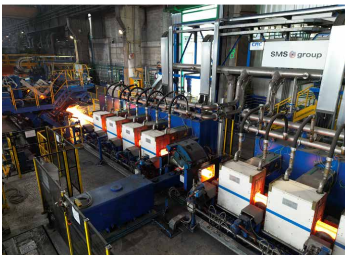
Feralpi Lonato stages 1 and 2 live pictures during production – December 2023: induction furnaces area (Picture: SMS group)
