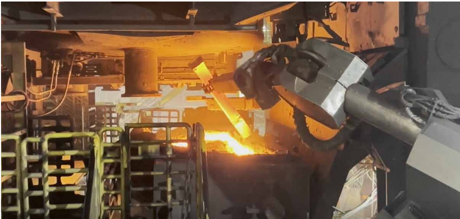
The new multitool robot operating at the casting machine under challenging operating conditions (Photo: Polytec)
