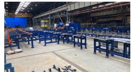
Parts of the new combination mill arriving at Tata Steel's Corby site (Picture: Tata Steel)
