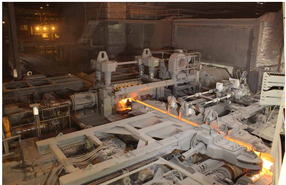
The blooming stand of the Imatra heavy bar mill will undergo a major revamp (Photo: Ovako)
