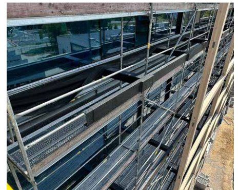
UPN sections in XCarb ® recycled and renewably produced are being installed in the balconies of the CD PROJEKT RED's new building in Warsaw (Photo: ArcelorMittal)
