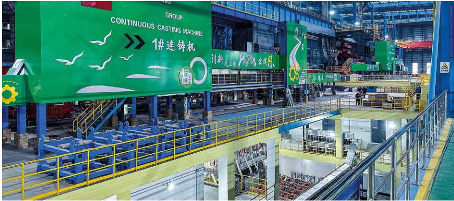
The newly equipped continuous casting shop at Jiangsu Yonggang (Photo: Danieli)
